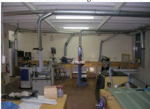
A Very impressive setup - note the dust extraction system
